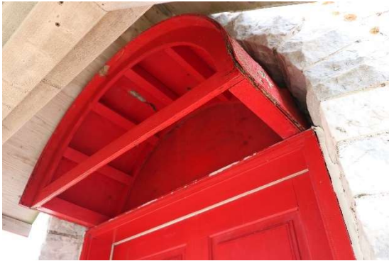
Figure 22: Support structure of the semi-circular stone facing to be redone and integrated with the new louver.
