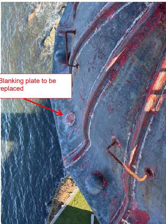
Figure 6 : Blanking plate to be replaced
