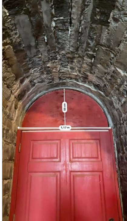
Figure 21: Estimated size of space for the integration of the new louver (1.17m x 0.66m)
