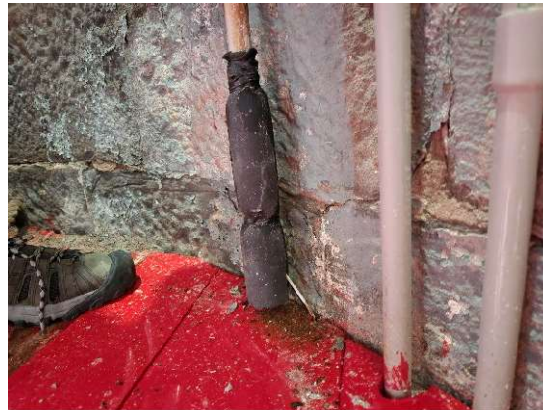
Figure 32: Broken electrical wire protector conduit to be repaired.
