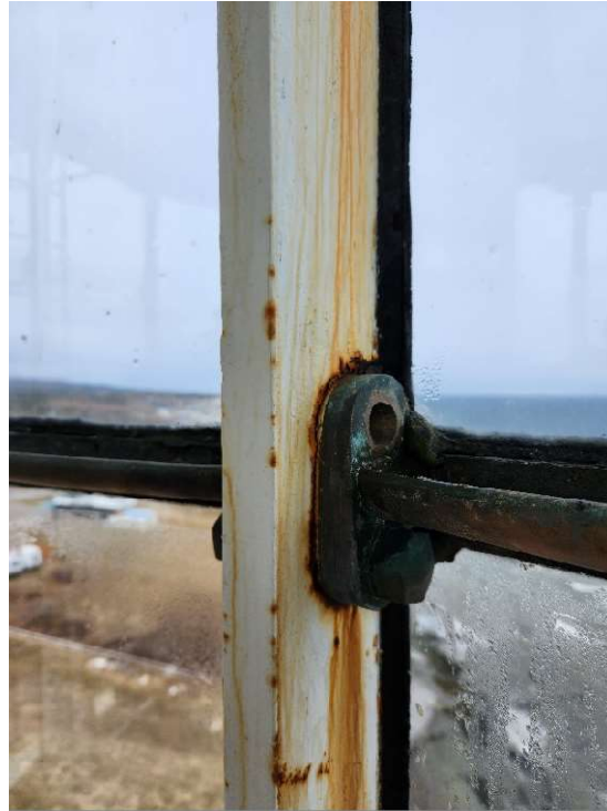
Figure 13: Missing bolts at some junctions between horizontal ties and structural vertical studs
