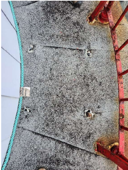
Figure 27: Obsolete anchors to be removed
