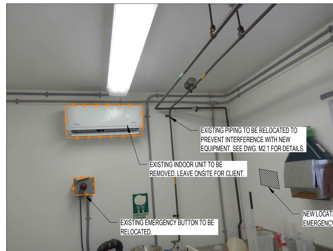
IMAGE #2: EXISTING FAN COIL INDOOR UNIT
