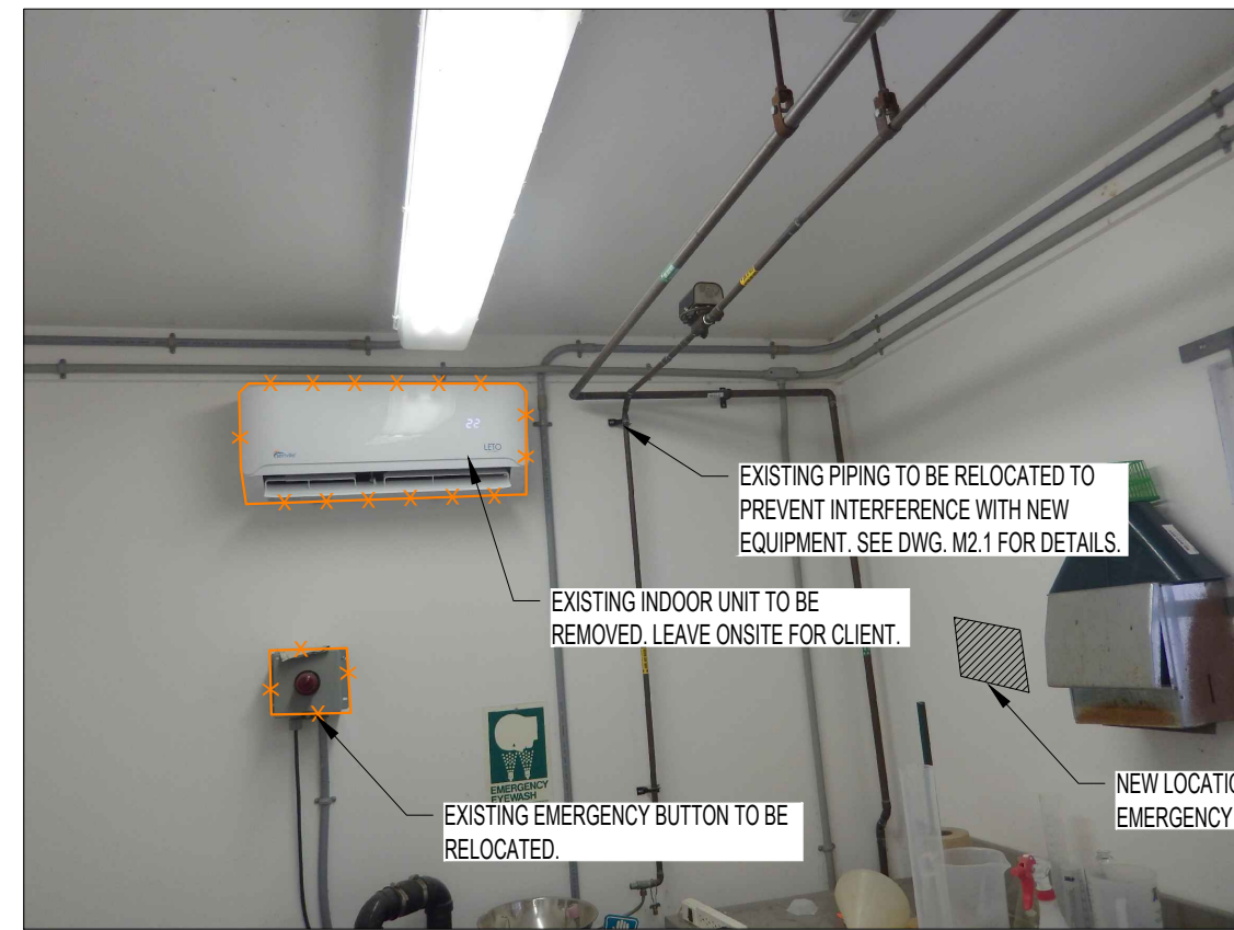
IMAGE #2: EXISTING FAN COIL INDOOR UNIT
