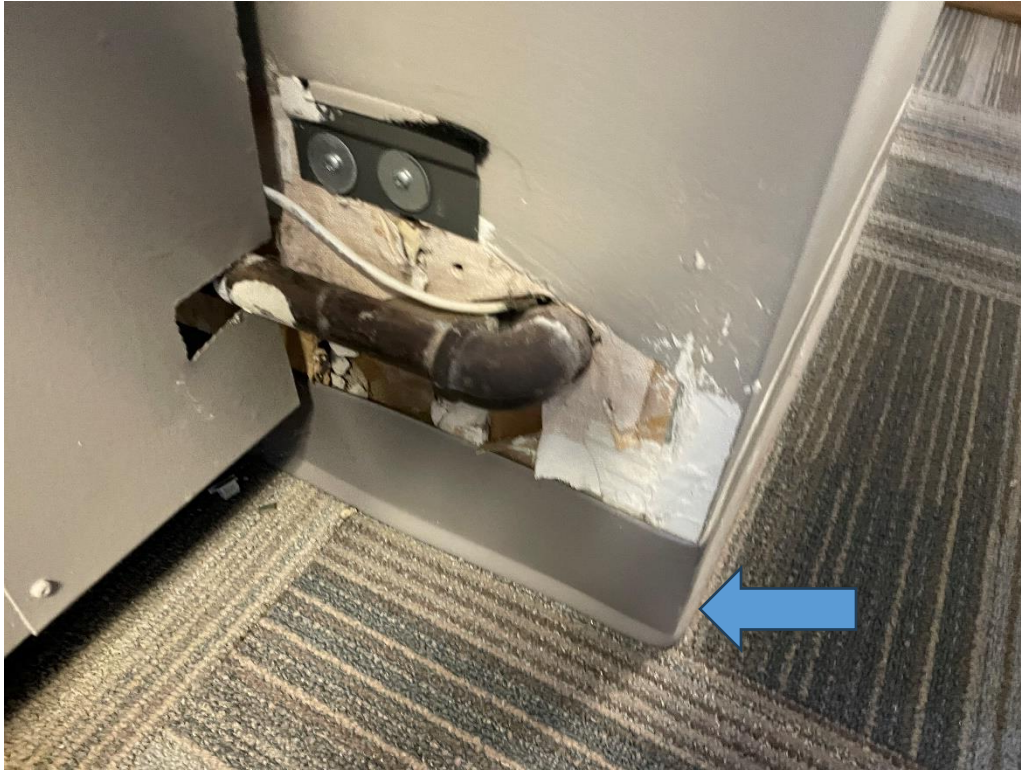
Figure 6: Representative photograph of non-asbestos containing vinyl baseboard/mastic observed throughout the project areas (Sample ID: AS-07A-C). Gray wall paint was also sampled from this location and is confirmed to be non-lead containing (Sample ID: LP-01, 8ppm).
