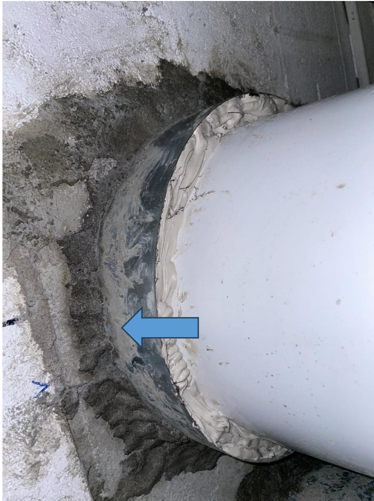
Figure 1: Representative photograph of non-asbestos containing cement parging at pipe penetrations within the Ground Floor Mechanical Room (Room 1457). Cement parging is confirmed to be non-asbestos containing (Sample ID: AS-01A-C)
