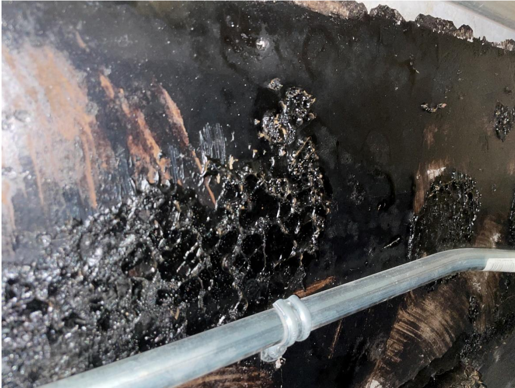
Figure 2: Representative photograph of non-asbestos containing black tar on cork board observed within the 2nd Floor ceiling space (Sample ID: AS-02A-C).
