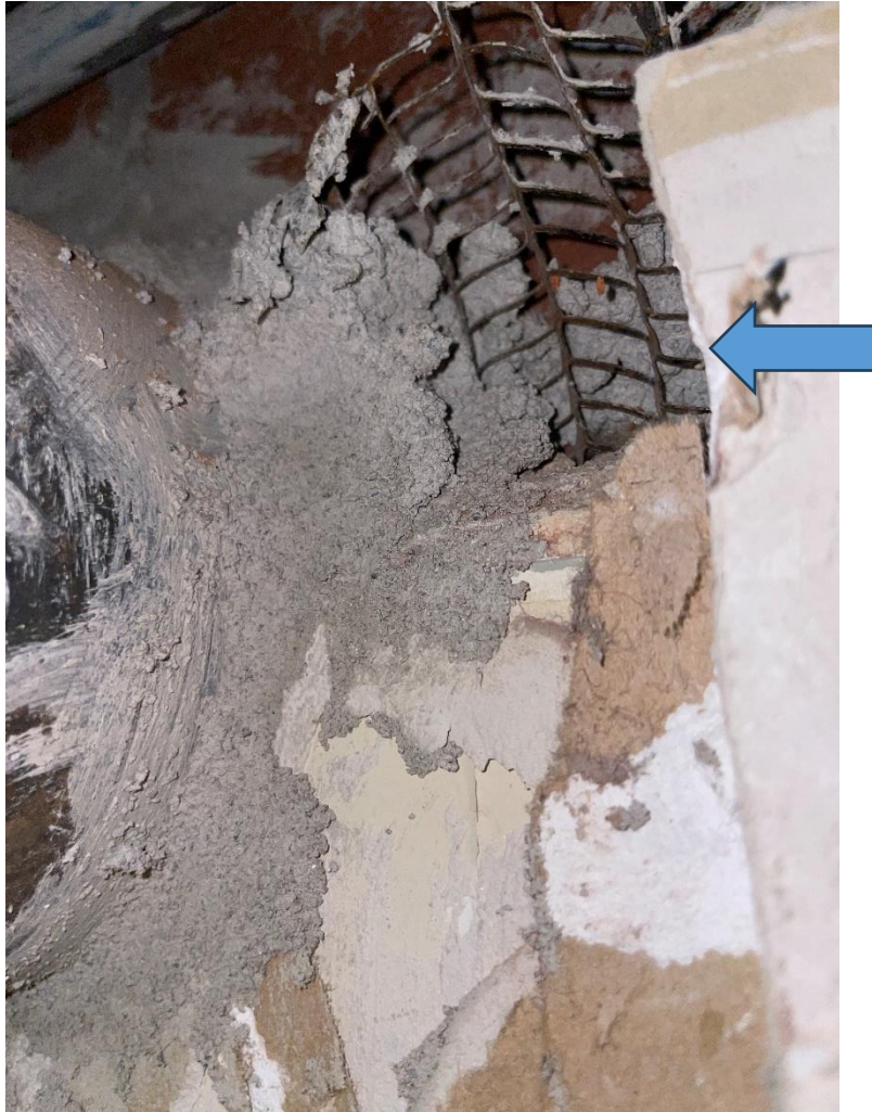
Figure 3: Representative photograph of wall plaster (white and gray layers) observed behind drywall throughout the project areas. Drywall joint compound is confirmed to be non-asbestos (Sample ID: AS-03A-D).
