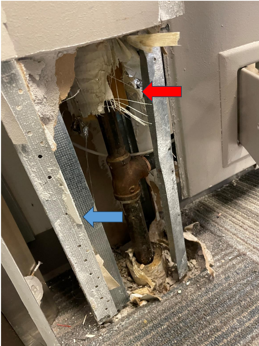
Figure 4: Representative photograph of drywall joint compound (blue arrow) observed in "Poor Condition" on the 2nd Floor at pipe penetrations. Drywall joint compound was sampled and confirmed to be non-asbestos containing (Sample ID: AS-04A-C). Fibreglass insulation (red arrow) was sampled as per client request and confirmed to be non-asbestos containing (Sample ID: AS-06A-C).
