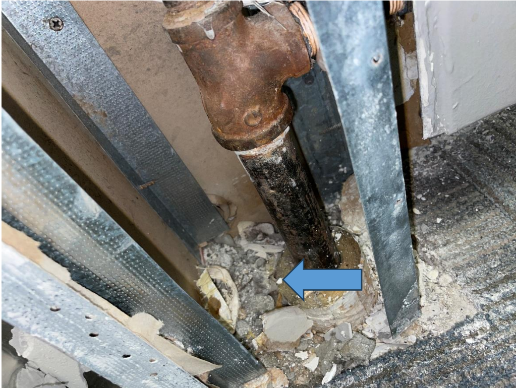
Figure 5: Representative photograph of cementitious debris observed at pipe penetrations on the 2 nd Floor adjacent to the Kitchen. The cementitious debris was sampled and confirmed to be non-asbestos containing (Sample ID: AS-05A-C).
