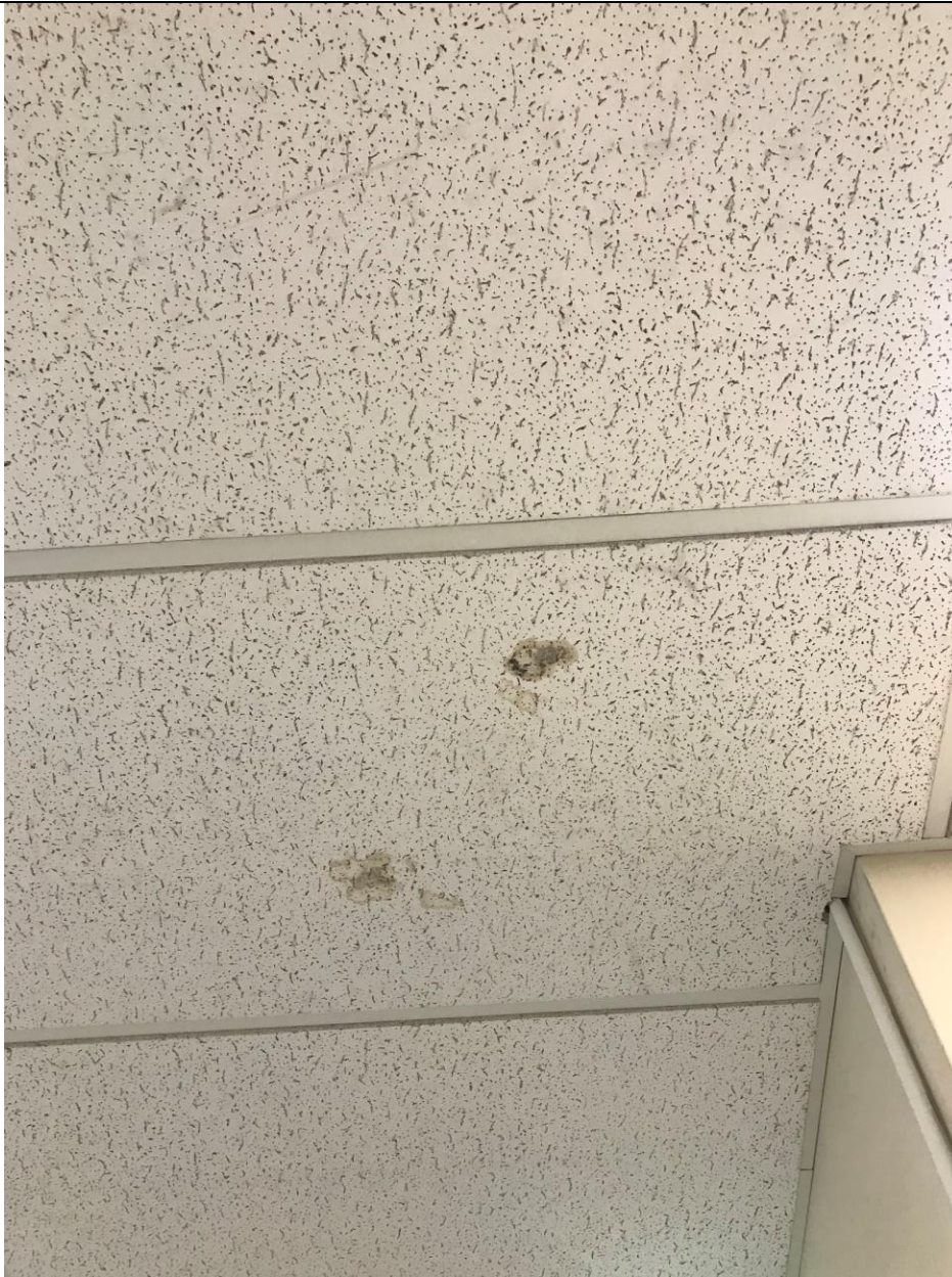
Photo 6: Suspected mould observed on ceiling tiles in room 152.
