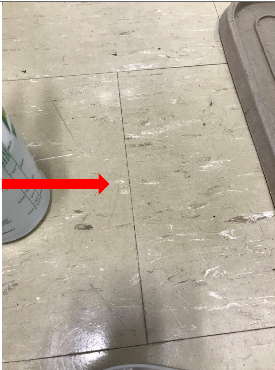
Photo 1: 12" x 12" vinyl floor tiles – tan with white streaks observed throughout the project area was confirmed to contain 3% Chrysotile asbestos (Englobe Sample ID 9698-01).
