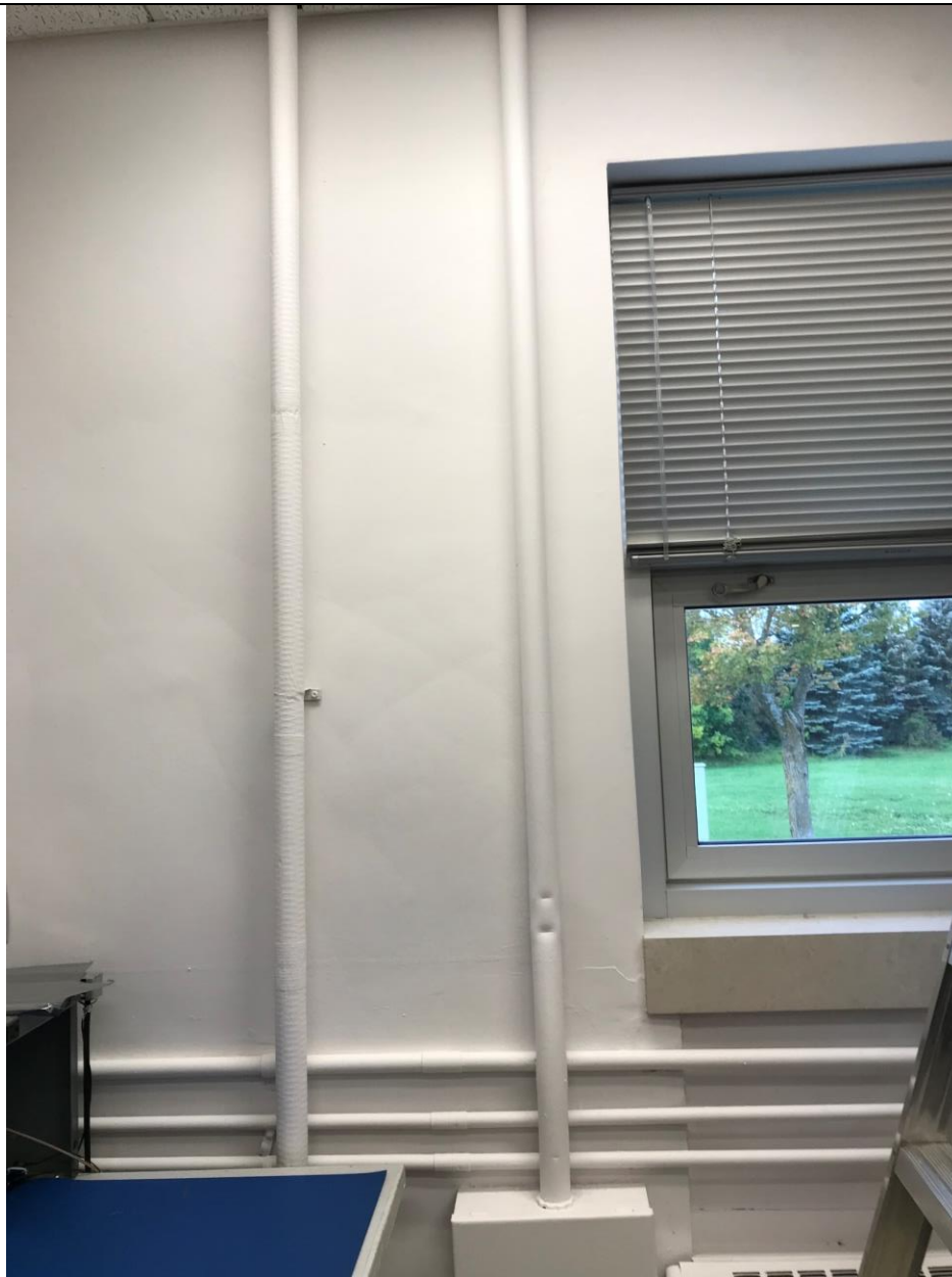
Photo 5: White wall paint observed in the back offices contains 388 ppm lead (Englobe Sample ID LP01).
