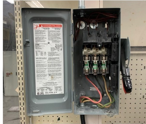
575 VAC / 3 Phase / 60 Hz, 30 amps power supply
