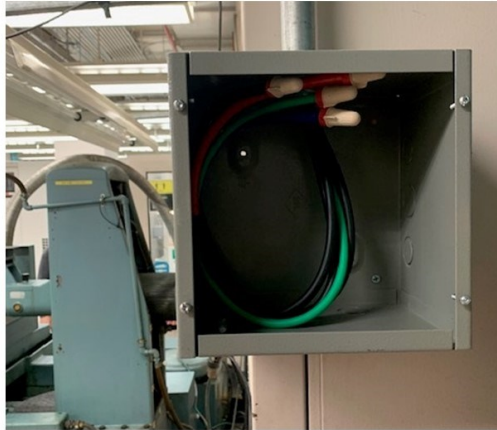
208 VAC / 3 Phase / 60 Hz, 70 amps power supply
