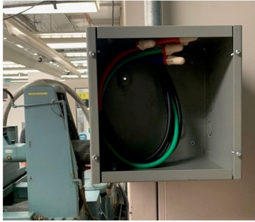
208 VAC / 3 Phase / 60 Hz, 70 amps power supply
