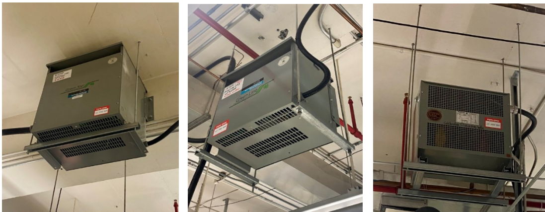
Figure 3-4 Examples of Installed Transformers Hanging from the Workshop Ceiling
