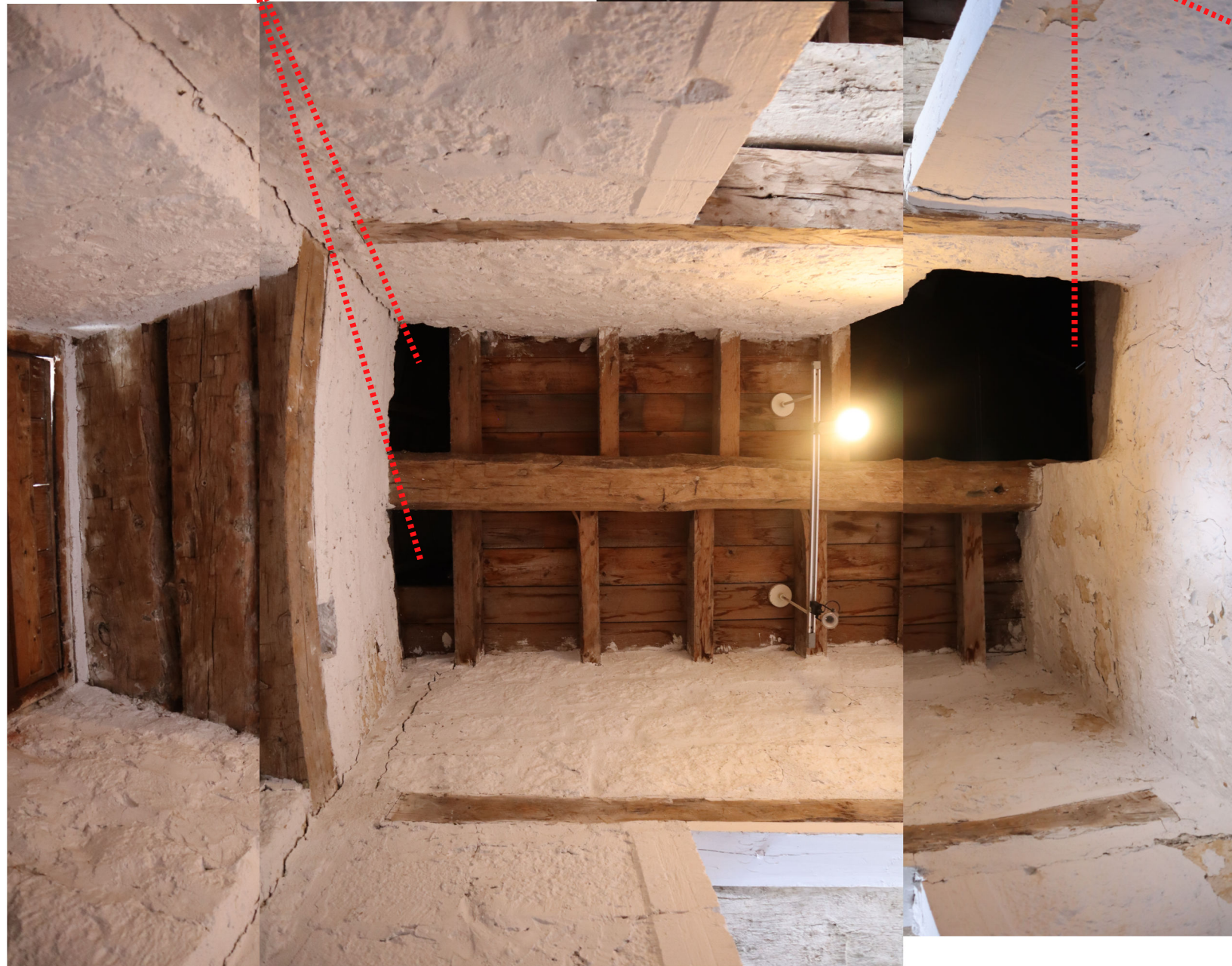
CEILING GAPS OPEN TO ATTIC
