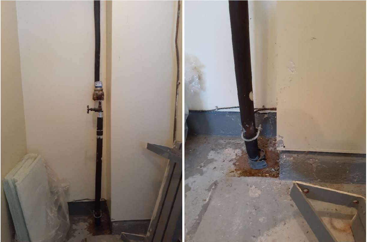
Figure 2: Representative photographs of the project area in the Mechanical Room in Building 129. Non-asbestos containing drywall joint compound located on the wall [Sample ID: 129-AS-01A-C]. Grey paint on the floor [ Sample ID: 129-LP-01; 458 ppm lead ] confirmed to contain higher levels of lead, and the beige paint on the wall [Sample ID: 129-LP-02; 6 ppm lead] contains low levels of lead.
