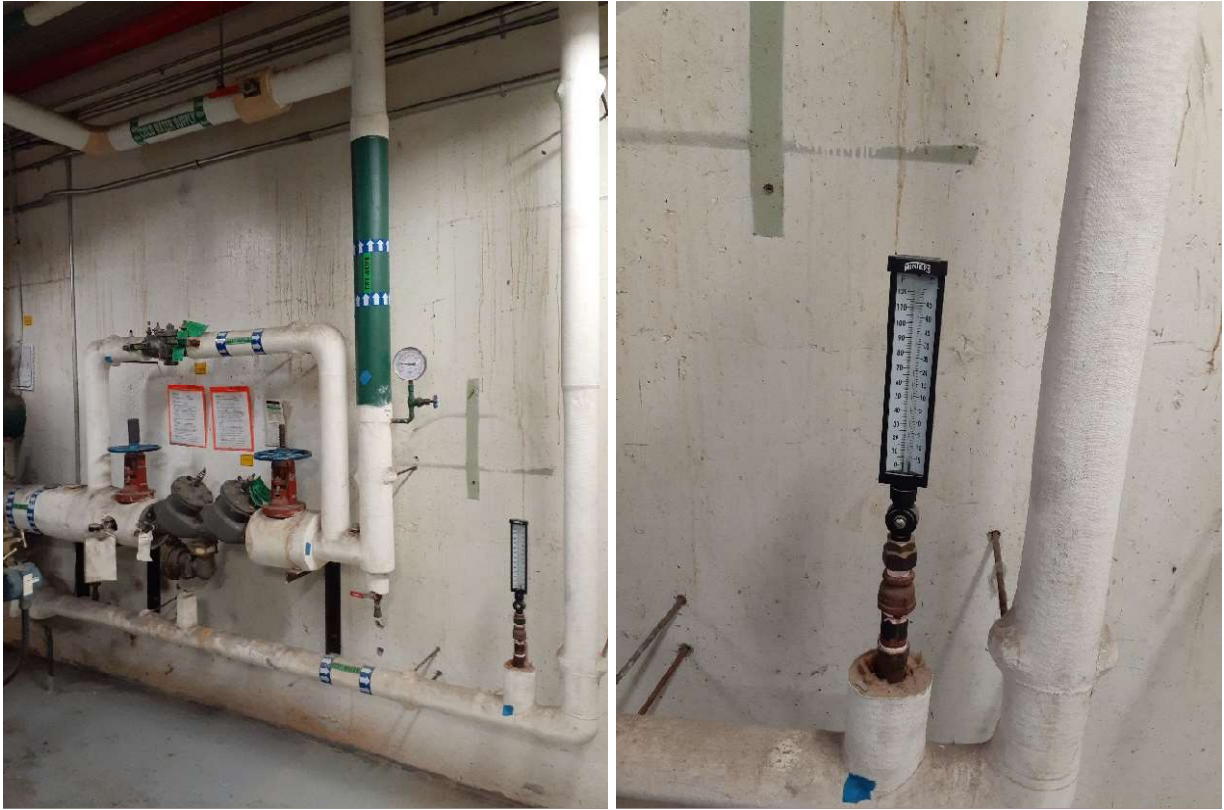
Figure 16: Representative photograph of the project area in the Mechanical Room of the Central Heating Plant. White paint on the wall [Sample ID: CHP-LP-02; 1,200 ppm lead] confirmed to contain higher levels of lead, and the grey paint on the floor [Sample ID: CHP-LP-01; 74 ppm lead] contains low levels of lead. Thermometer suspected to contain mercury . Pipe insulation in the project area confirmed to be non asbestos containing.
