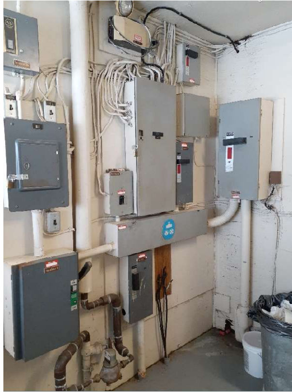
Figure 14: Representative photograph of the project area in the Office Space of Building 220. Grey paint on the floor [ Sample ID: 220-LP-02; 566 ppm lead ] confirmed to contain higher levels of lead, and the beige paint on the wall [Sample ID: 220-LP-01; 8 ppm lead] contains low levels of lead.
