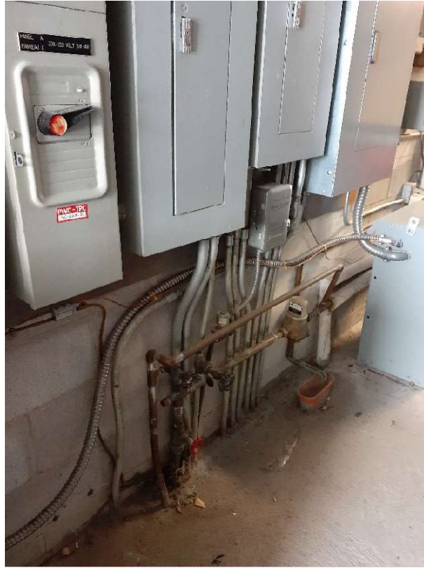
Figure 13: Representative photograph of the project area in the Mechanical Room in Building 211. Grey paint on the floor [Sample ID: 211-LP-01; 2,250 ppm lead] confirmed to contain high levels of lead.
