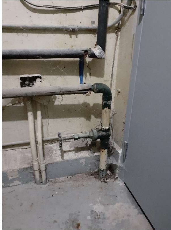
Figure 1: Representative photograph of the project area in the Mechanical Room in Building 128. Grey paint on the floor [Sample ID: 128-LP-01; 1,460 ppm lead] and beige paint on the wall [Sample ID: 128-LP-02; 1,010 ppm lead] confirmed to contain high levels of lead. Pipe insulation observed to be non asbestos containing foam.
