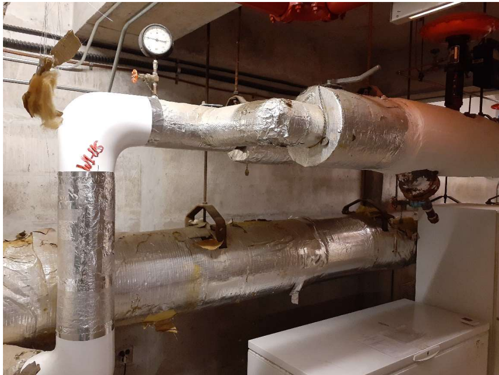
Figure 9: Representative photograph of the project area in the Mechanical Room in the C-Wing of Building 201. Tar paper under fibreglass insulation was confirmed to be non asbestos containing – 201-AS-01A-C.
