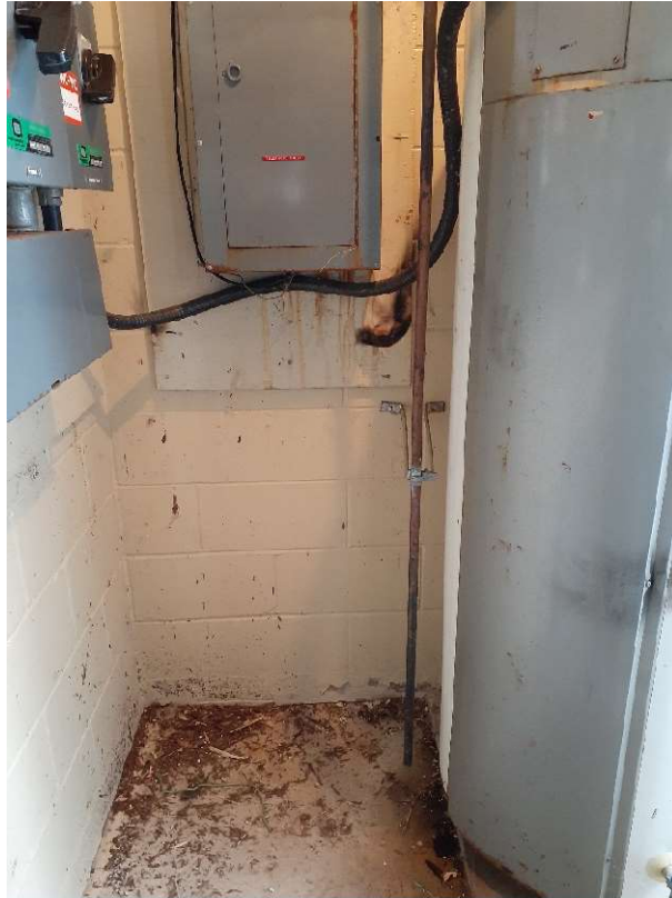
Figure 8: Representative photograph of the Mechanical Room in Building 169. Non-asbestos containing concrete block mortar located on the wall [Sample ID: 169-AS-01A-C]. Beige paint on the wall [Sample ID: 169-LP-01; 41 ppm lead] contains low levels of lead.
