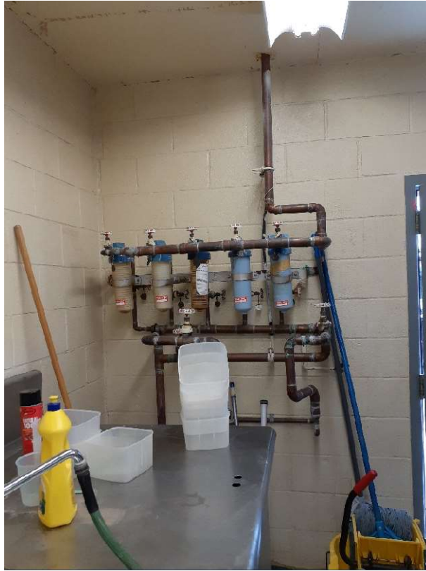
Figure 12: Representative photograph of the project area in the Seed Storage Room in Building 210. Non-asbestos containing concrete block mortar located on the wall [Sample ID: 210-AS-01A-C]. Beige paint on the wall [Sample ID: 210-LP-01; 12 ppm lead] contains low levels of lead.
