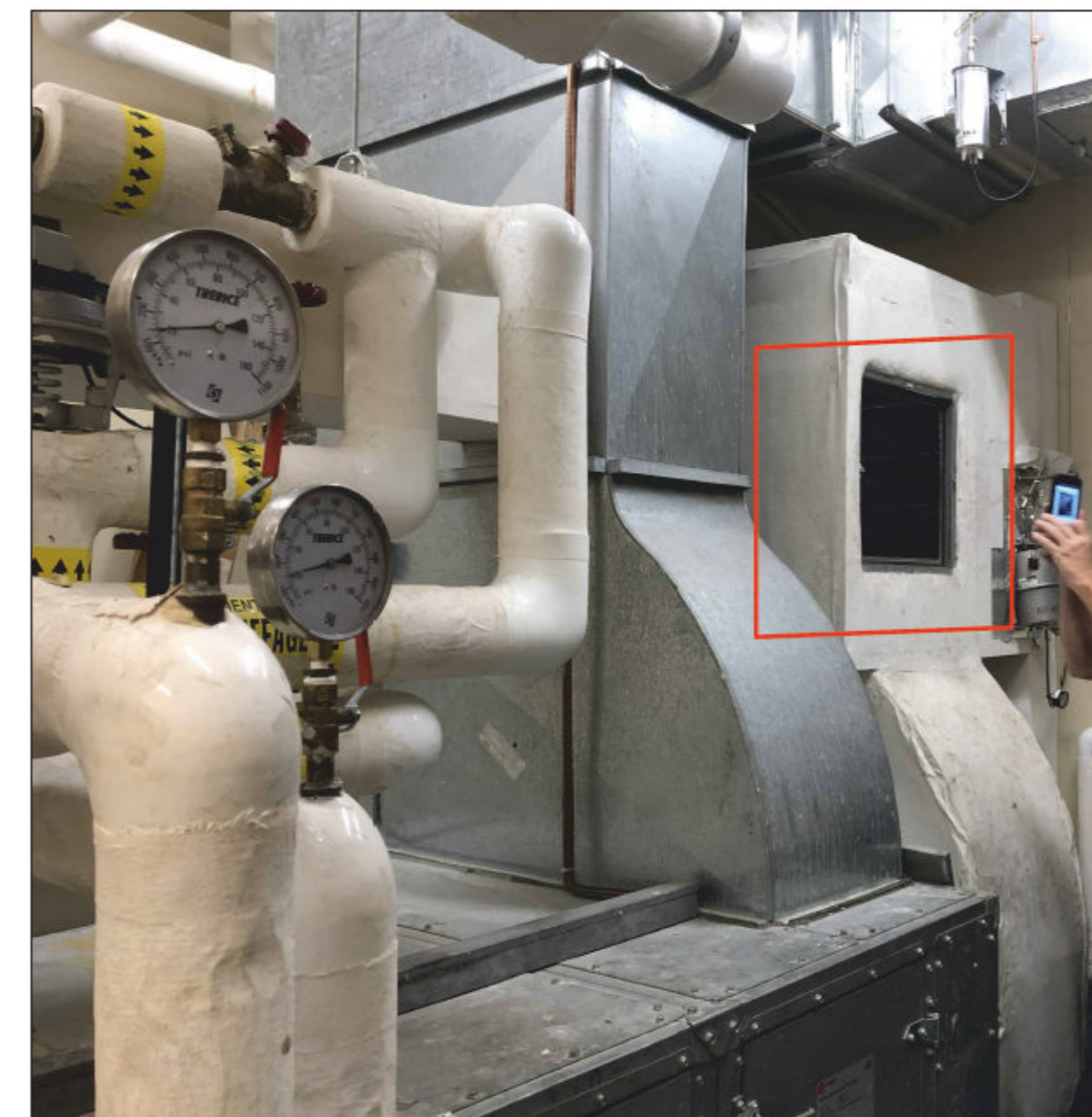
LOCATION OF MOTORIZED DAMPER
