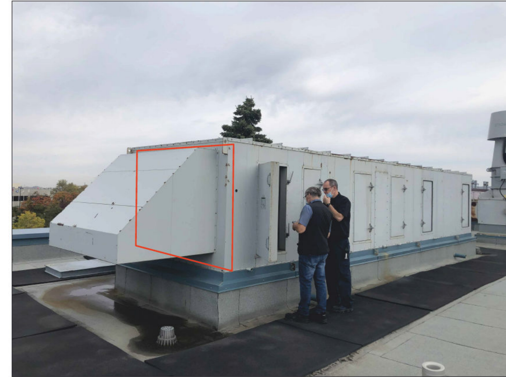
LOCATION OF MOTORIZED DAMPER
