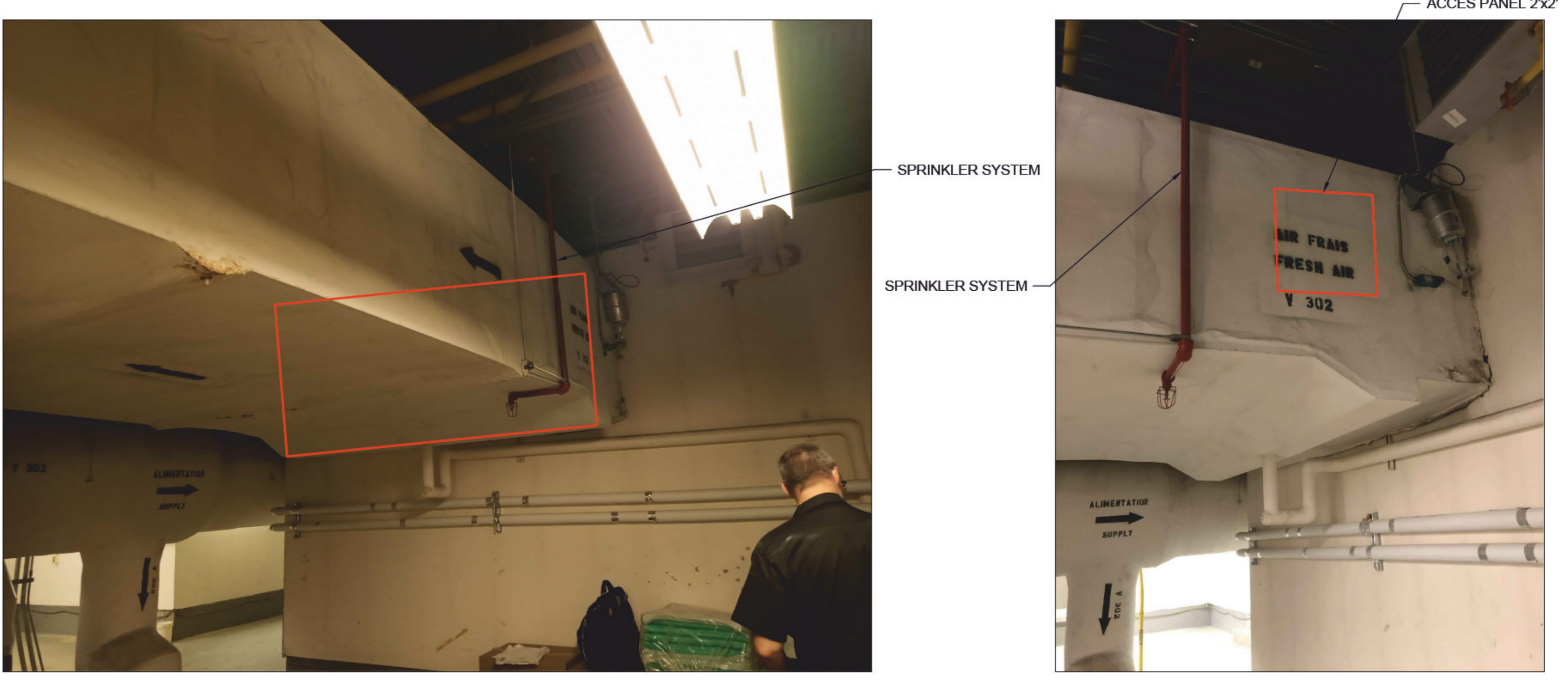
LOCATION OF MOTORIZED DAMPER
