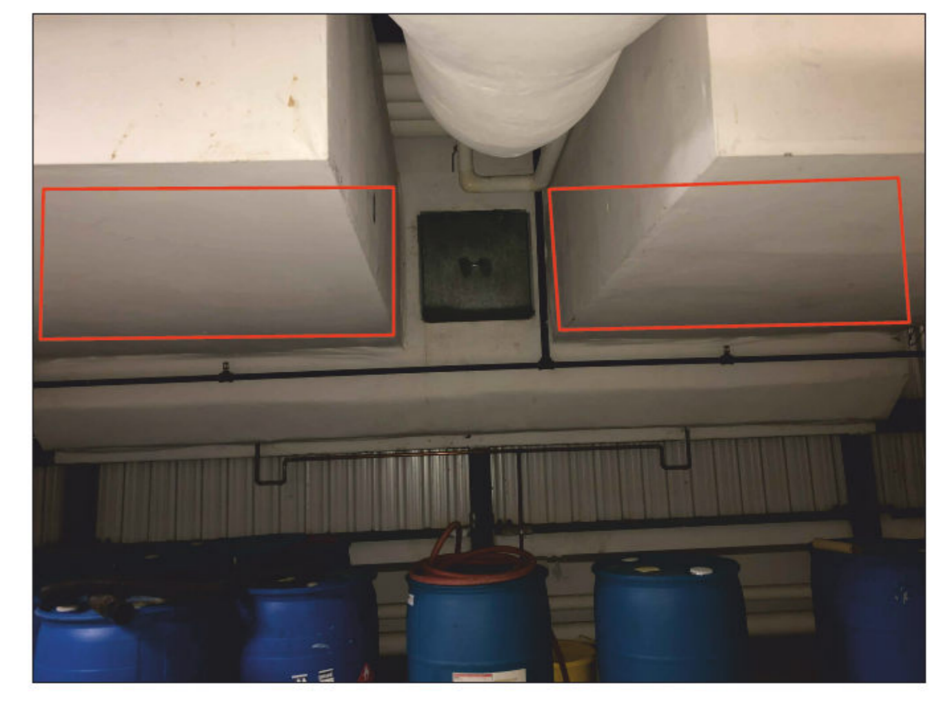
LOCATION OF MOTORIZED DAMPER
