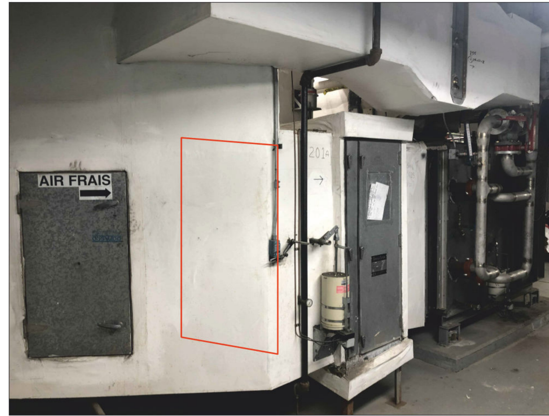
LOCATION OF MOTORIZED DAMPER
