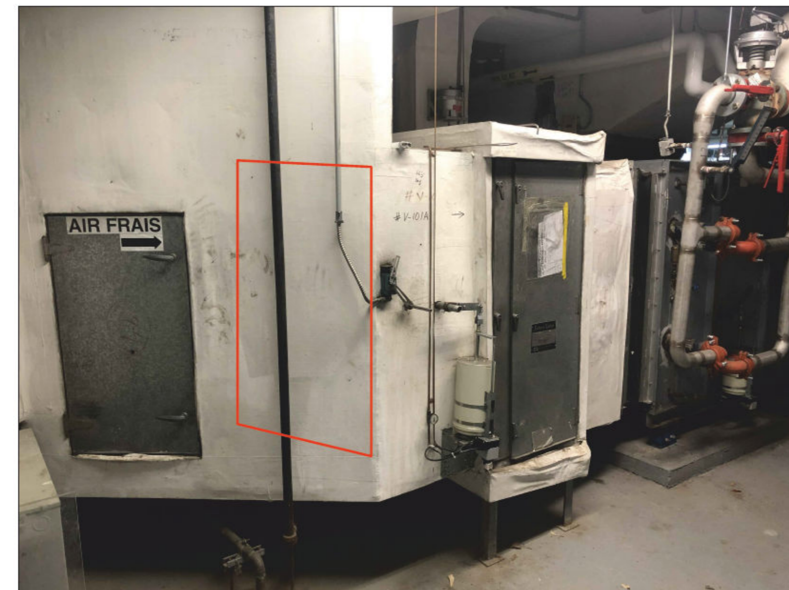
LOCATION OF MOTORIZED DAMPER
